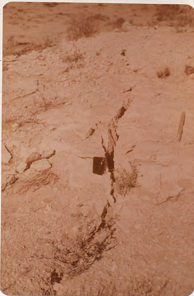
Figure A1-14. Fissure cutting through hard caliche north of Cheyenne Road, section 10ddc, T20S-R61E.
