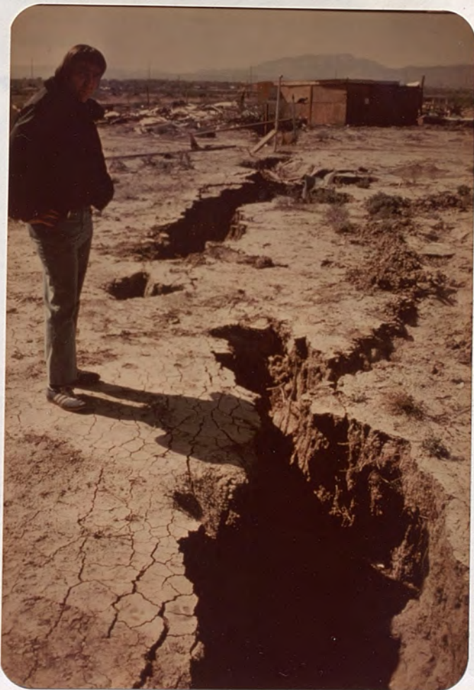
Figure A1-16. Fissure developed during and after flash flood event west of Simmons Road, section 18d, T20S-R61E.
