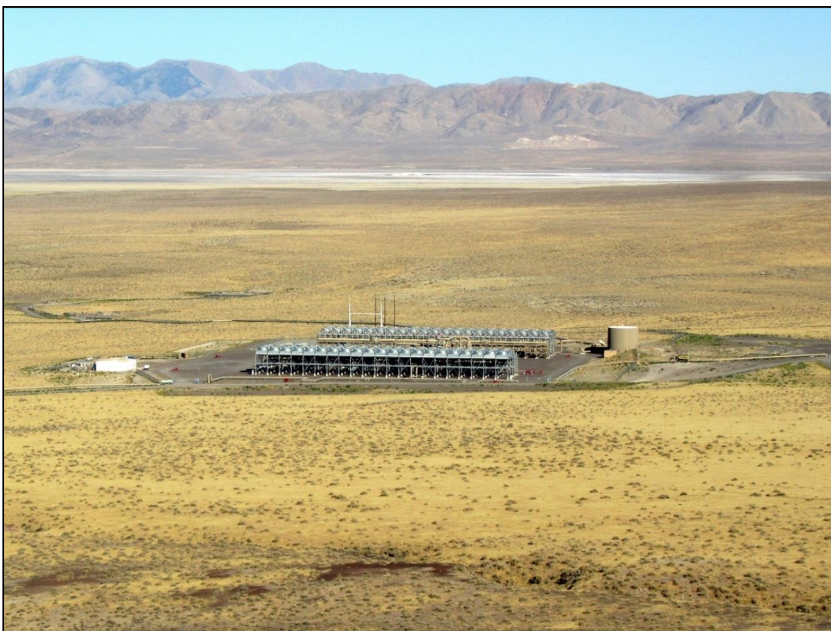
Figure 12. Photo of the 13.4 MWe capacity binary power plant at the Salt Wells geothermal area (figure 11). Photo by Nicholas Hinz, 2011.
